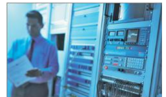
Headend/Central Office/ Hubs/OSP
